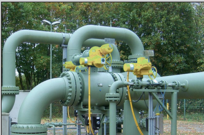
Typical gas-oriented application with x-matic actuators mounted on ball valves
